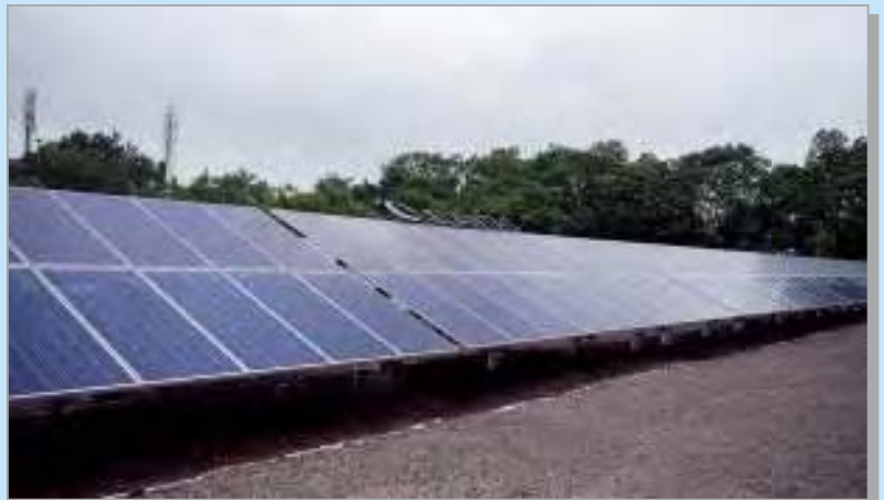
Solar photovoltaic panels for the R & D Centre & Corporate office
