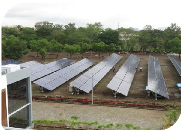
Solar panels - Pimpri Plant
