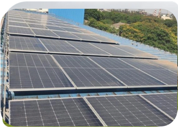
Rooftop solar panels - Ankleshwar Plant
